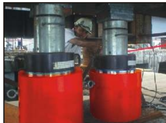
Single acting lock nut, load return cylinders used to support roof in a Tunnel Building project
