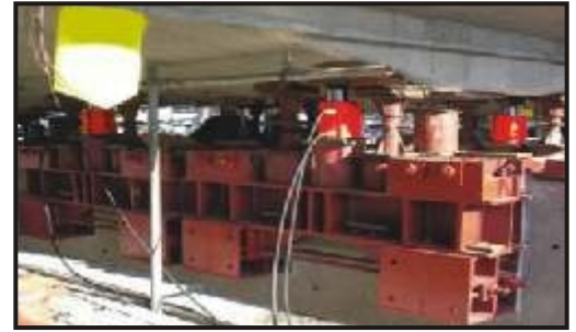
Double acting cylinder used for Bridge Lifting / Modification
