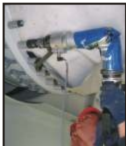
Bolting with angular (90°) electric nut runner where there is a space constraint
