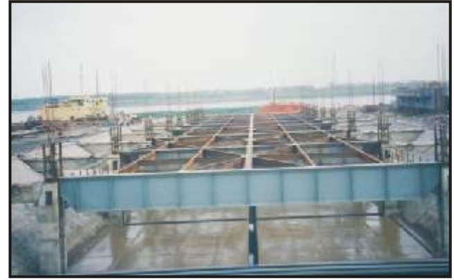
Ship Repair Platform / Manipulators with screwed ram lock nut cylinders
