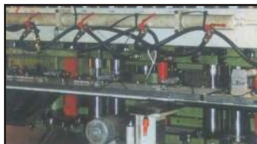
Cylinders used in Paper Mill for trimming
